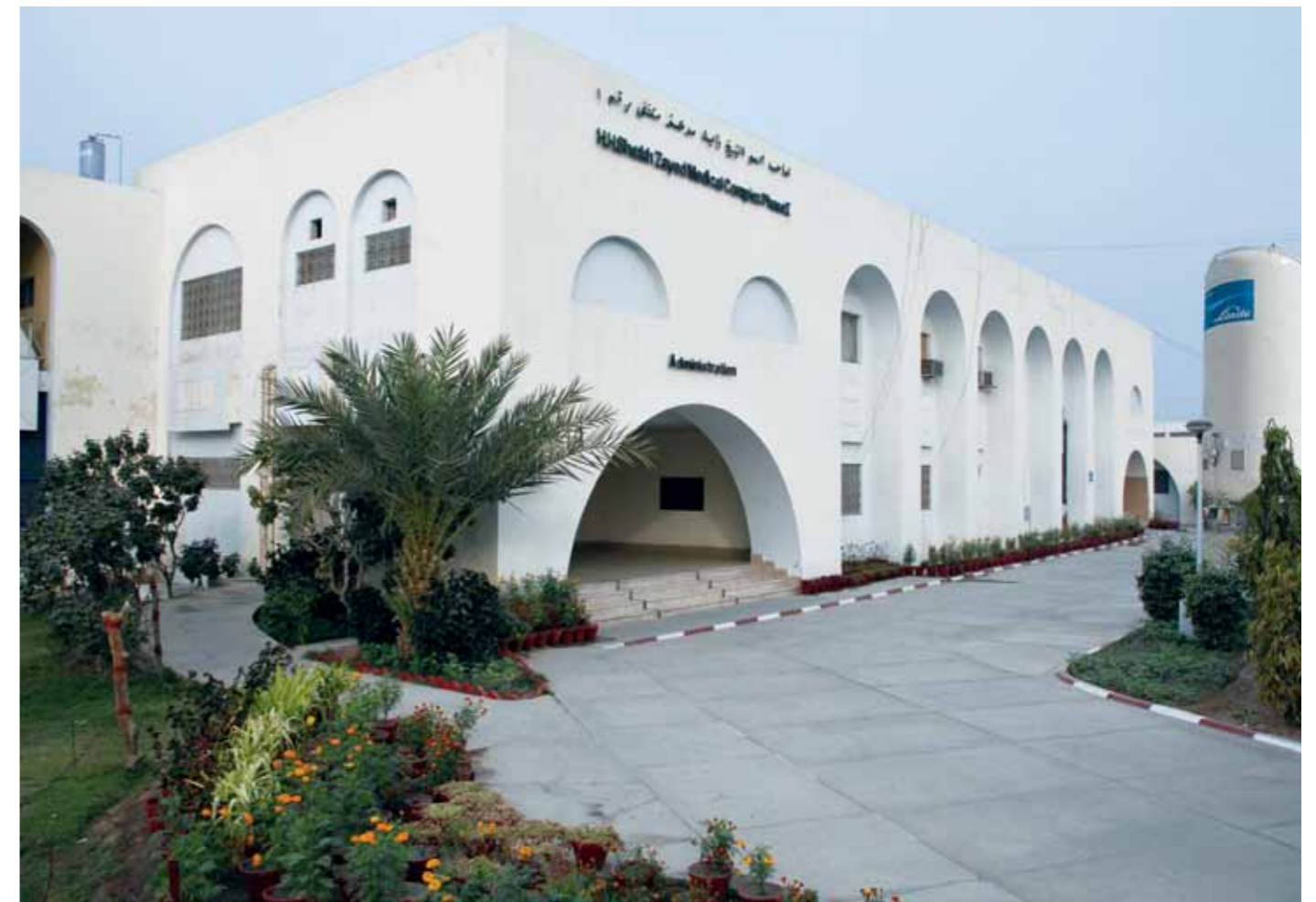
Linde installed a 10 KL tank for bulk liquid medical oxygen at Sheikh Zayed Medical College and Hospital, Rahim Yar Khan
