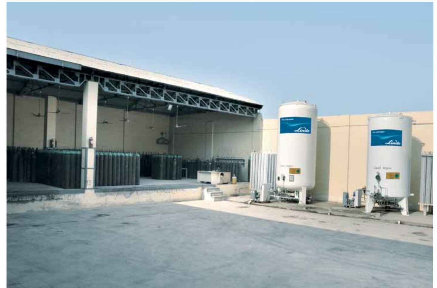
Expansion at a major customer site to capitalize growth in secondary cutting segment
